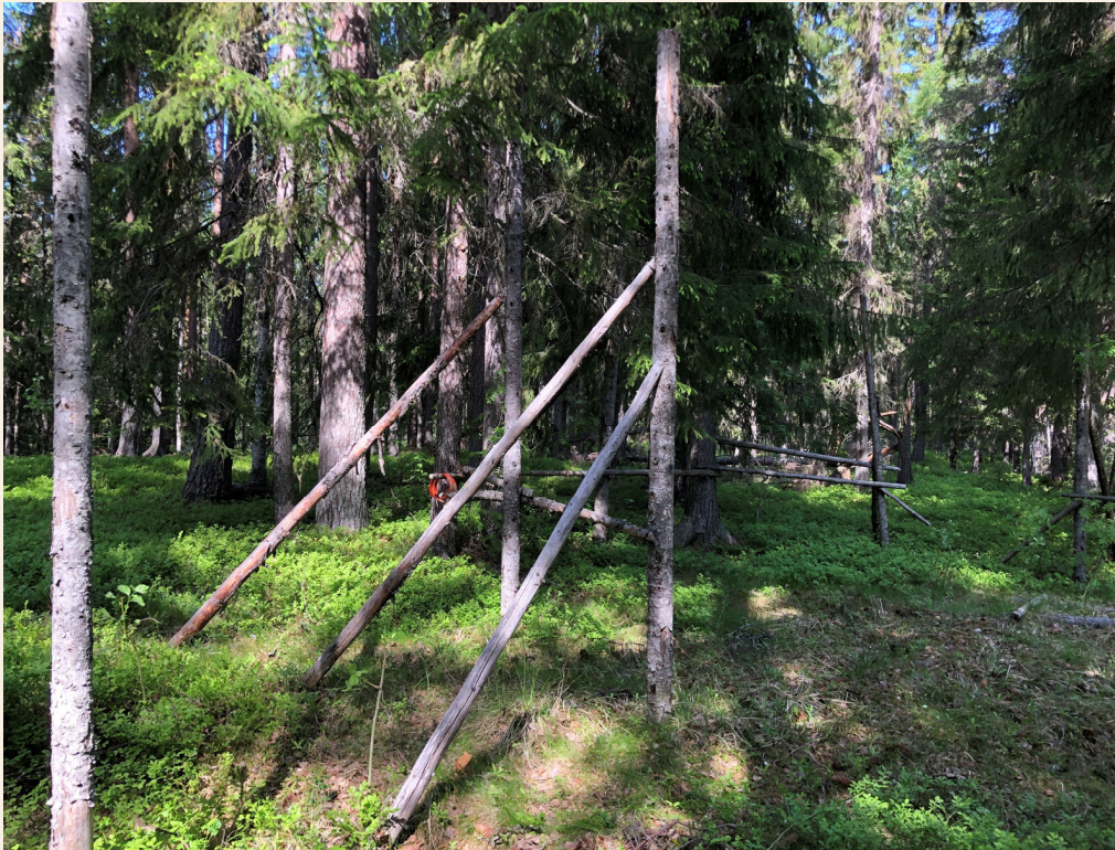
Work yard where the forest is to be thinned out according to the wishes of the Sami village. Collaborative planning was carried out in field summer of 2023. Photo: Anna Marntell ©.
