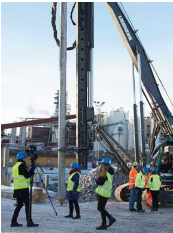
Work on the Östrand project began in February 2016 with a 12 meter concrete pile being driven into the ground.
